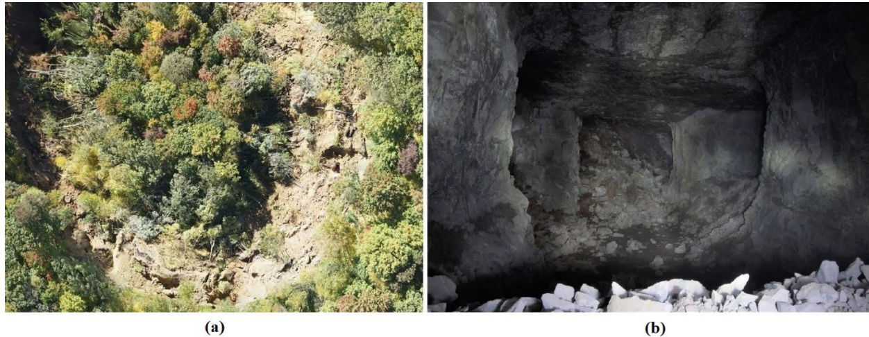
Figure 4. (a) Subsidence from collapsed workings and (b) an underground perspective of the rubblized periphery
