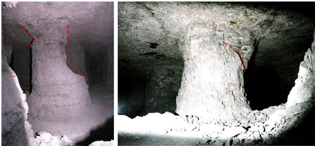
Figure 9. Pillars involved in the massive pillar collapse of Mine D (Photo credit: Dr. G.S. Esterhuizen)
