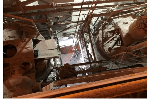
A contract employee, who was not wearing fall protection when a wooden board broke, fell 23 feet onto a concrete floor.
