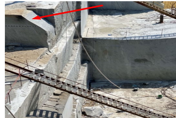
A miner was standing on a rock ledge when a triangular section of the rock broke, causing him to fall approximately 47 feet.
