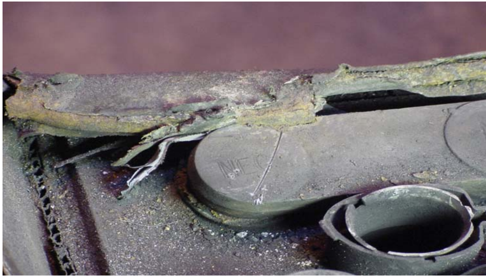
Scoop battery from under rock fall on 4 Section showing terminal contact with battery tray.
