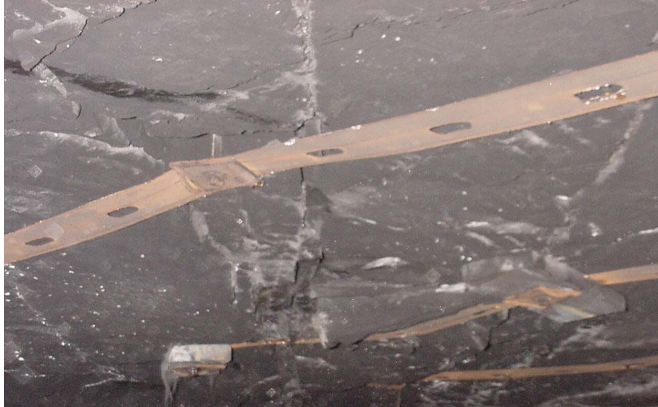
No. 2 Entry in 4 Section showing joints in mine roof .
