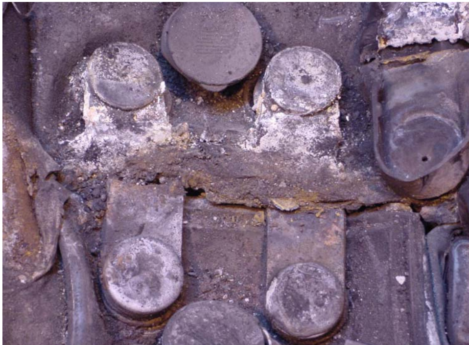
Scoop battery from under rock fall on 4 Section showing terminal damage.
