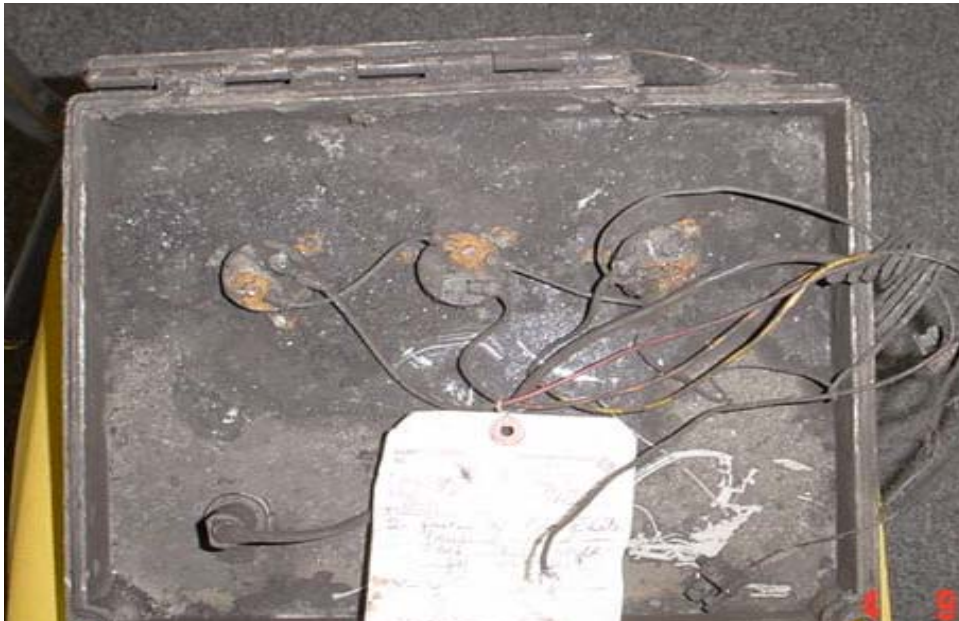
No. 4 Section track entry block light showing inside of block light.
