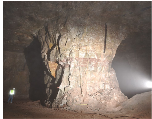
Fig. 7 Pillar affected by angular jointing adjacent to the collapsed area
