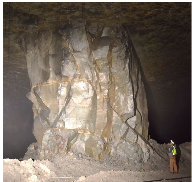
Fig. 4 Prominent N60°W striking joint intersecting a pillar south of the collapsed area
