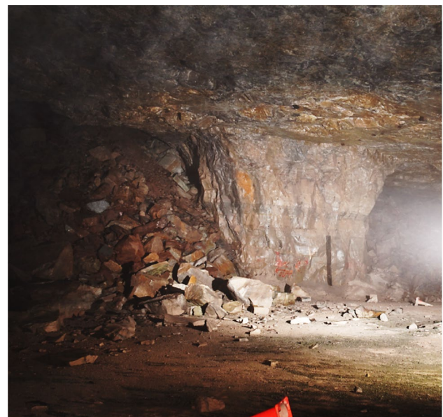
Fig. 8 Rubble from the roof collapse and a stable pillar along the edge of the area that collapsed
