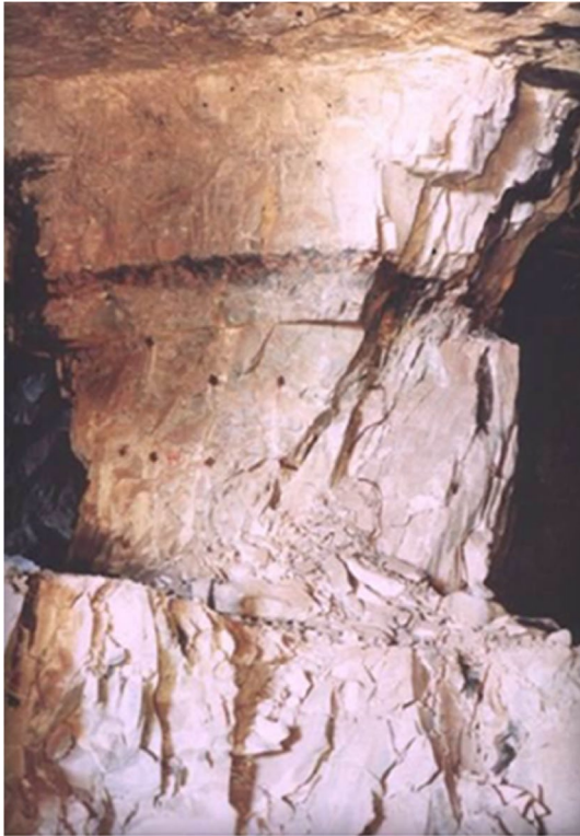
Fig. 6 Pillar impacted by large angular joints along the edge of bench mining showing sections of the pillar that fell away during bench mining (photo by A. T. Iannacchione)
