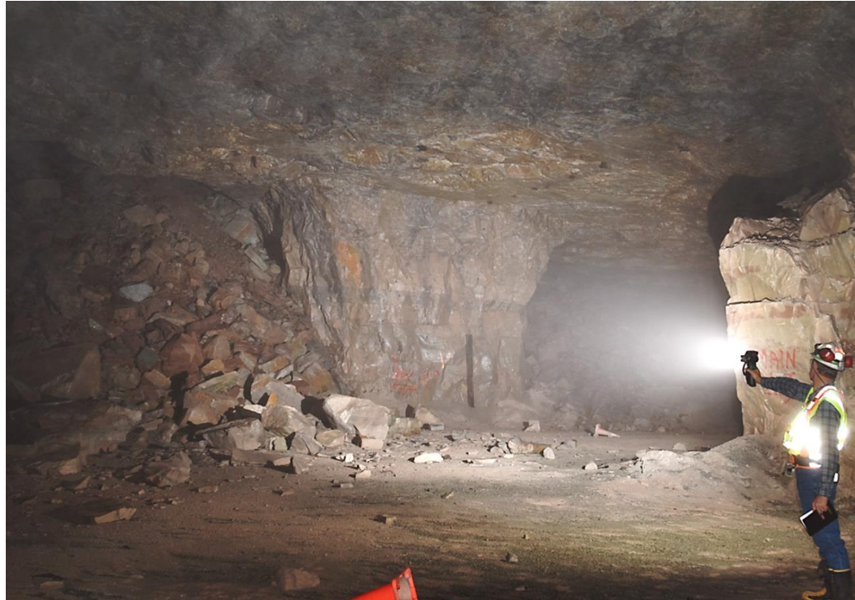
Edge of collapsed area near portal – mine in PA
