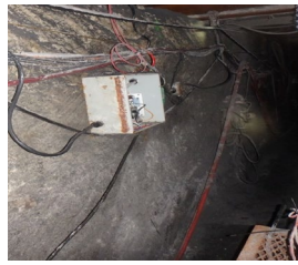
Work performed inside an energized enclosure.
