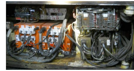
Open control panel exposing electrical connectors.
