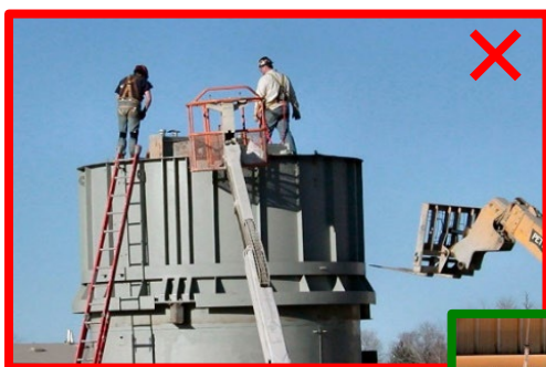
Above: Unsafe - No place to attach workers' lanyards
