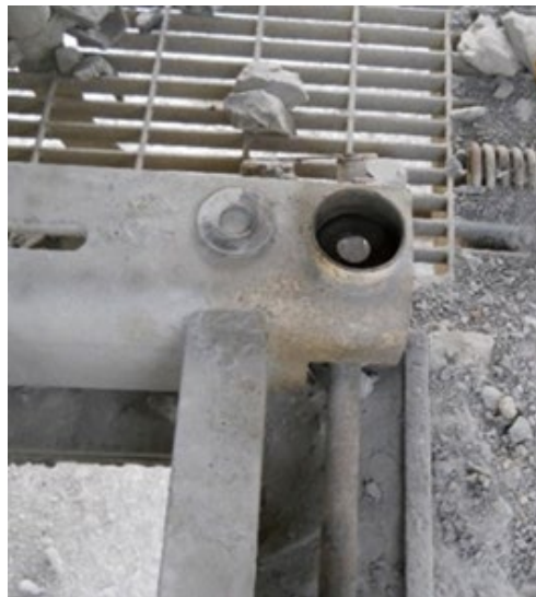
Broken Tension Bolt
