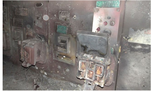
An electrician and trainee electrician were injured by an arc flash after the electrician re-entered a grounded cable into a cathead and energized the breaker.
