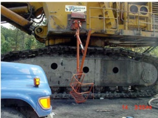
Figure 1: Failure of lift from improper welding
