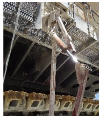
Figure 2: Failure of lift from undetected cracking
