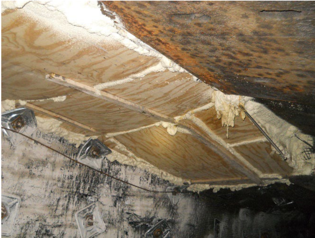
Improper application of a polyurethane-based foam product filling a high-volume void.
