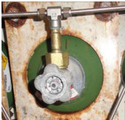
Figure 1 – View of Installed Fitting
