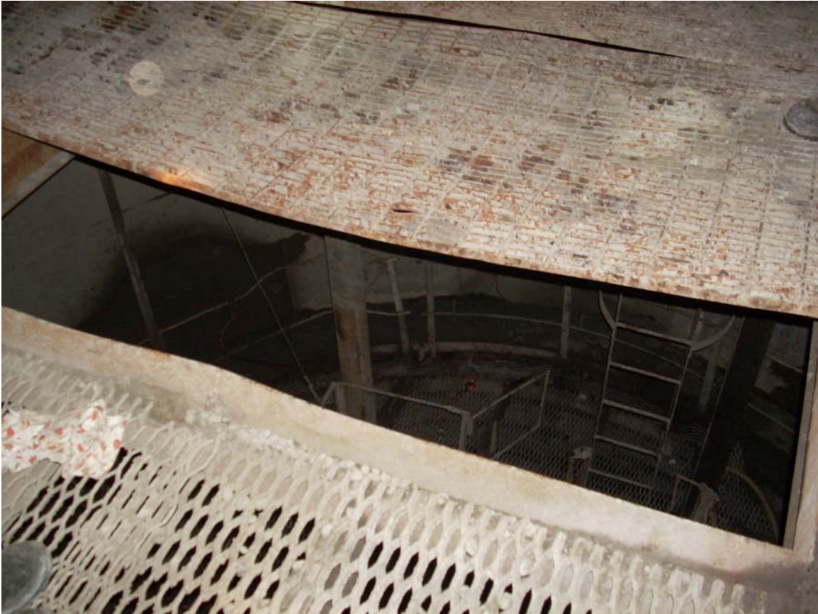
Photograph showing the top deck bucket well opening with one section of grating removed.
