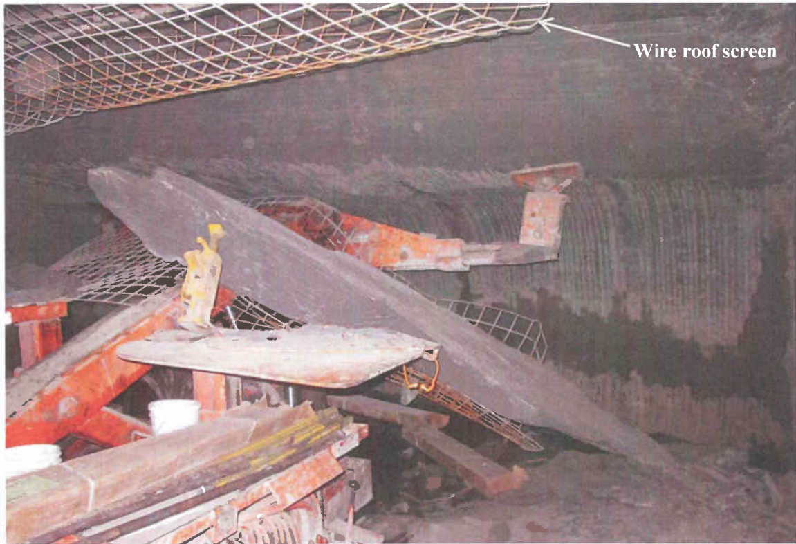
NUMBER 2 SLOPE ENTRY, APPROXIMATELY 170 FEET INBY SURVEY STATION NUMBER 4794 IN THE A MAINS SECTION
