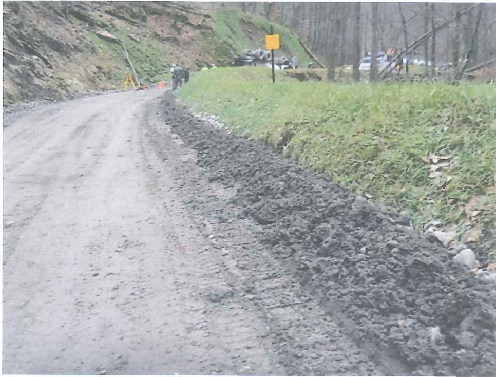
Close up view: Illustrating the condition of the Eagle Land haul road near the accident scene
