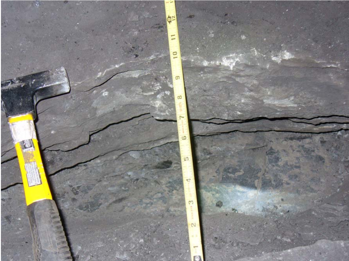
Figure Q-6. View of exposed floor heave crack looking straight down, with hammer and tape measure for scale. The crack is rootless and dies out approximately 12 inches into the floor at a layer of shale.
