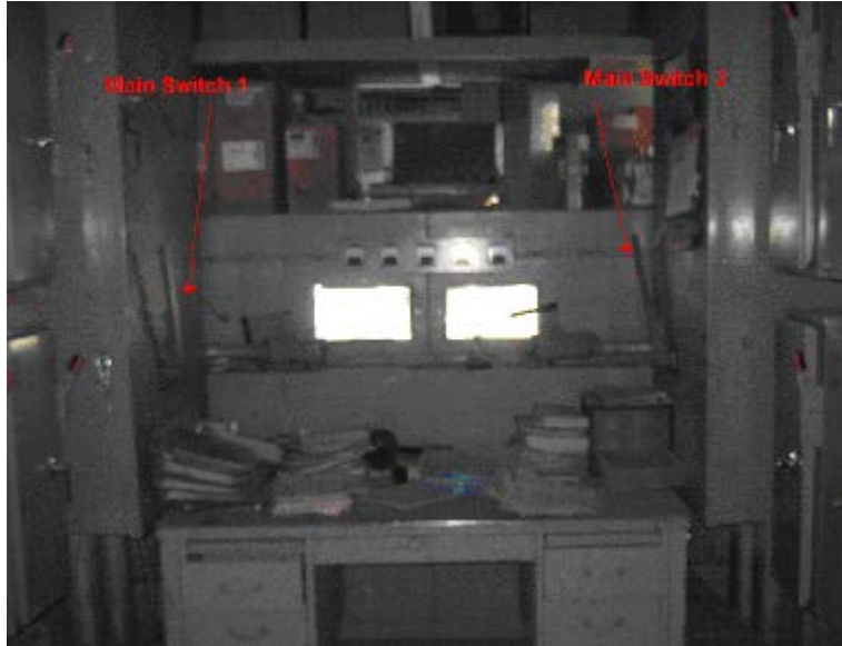
Main Switches Located Inside MCC
