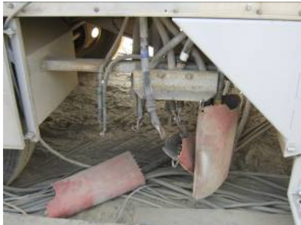
Power Entrance Line Side 2
