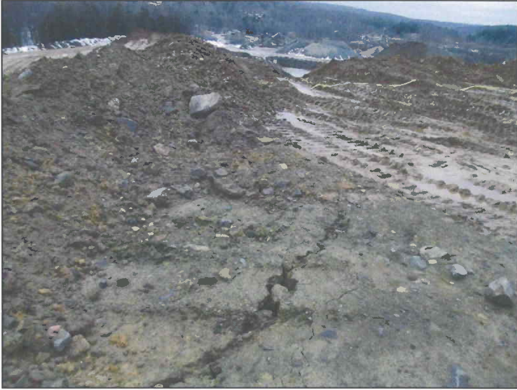
Figure 11 - Cracking observed on the surface of the dump.
