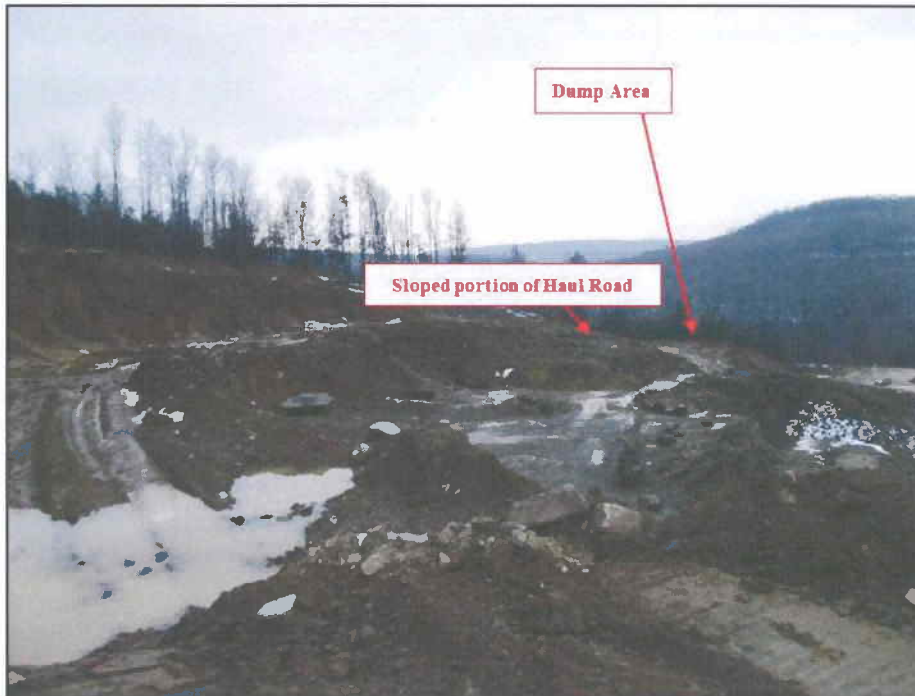
Figure 3 - Haulage route to dump location where the accident occurred.
