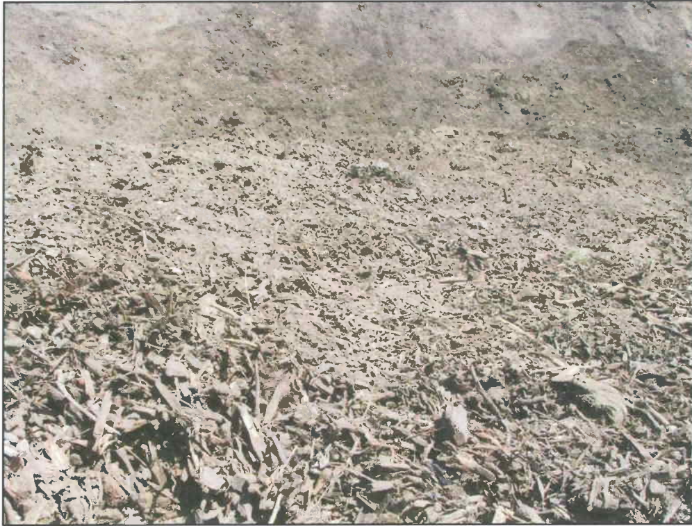
Figure 4 – Close-up view of failed backfill material composed of loam and mulch.
