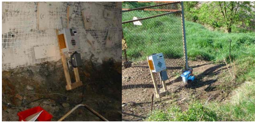
Figure 27: Transtek Telemag Unit; Underground and Surface @ 270'
